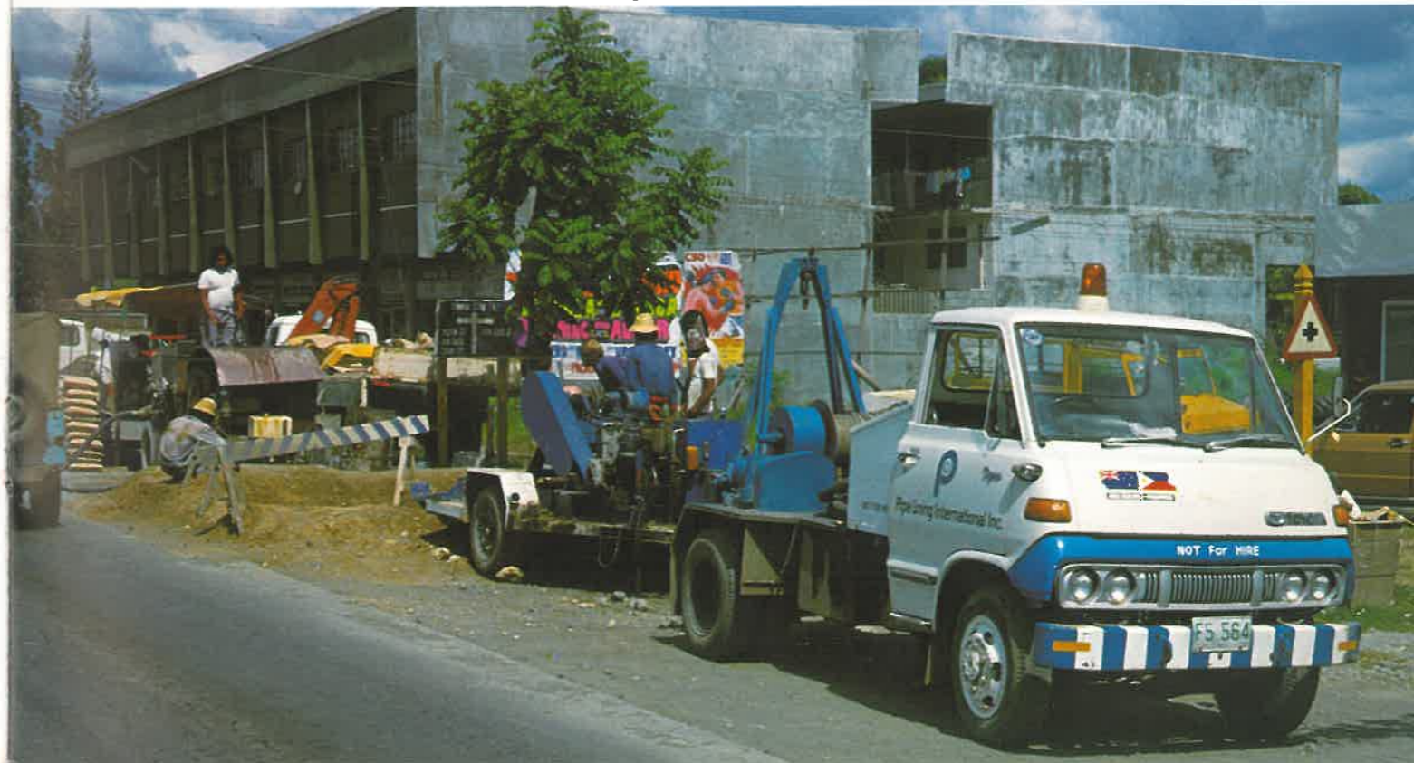
BELOW: In-situ cleaning and re-lining of watermains and sewer pipes is conducted in the Philippines by joint venture company, Pipelining International Ltd.
